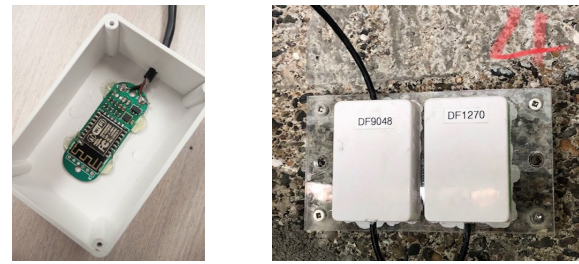
Fig. 4. Photo (a) shows the tilt sensor before being encased in waterproof resin. Photo (b) shows sensor "cluster 4" on the seawall.
